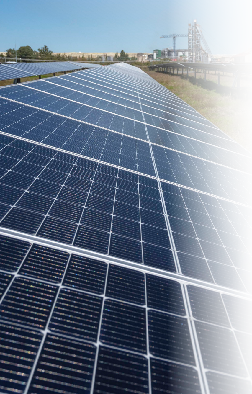
Evander Mines' 9.9MW solar plant
