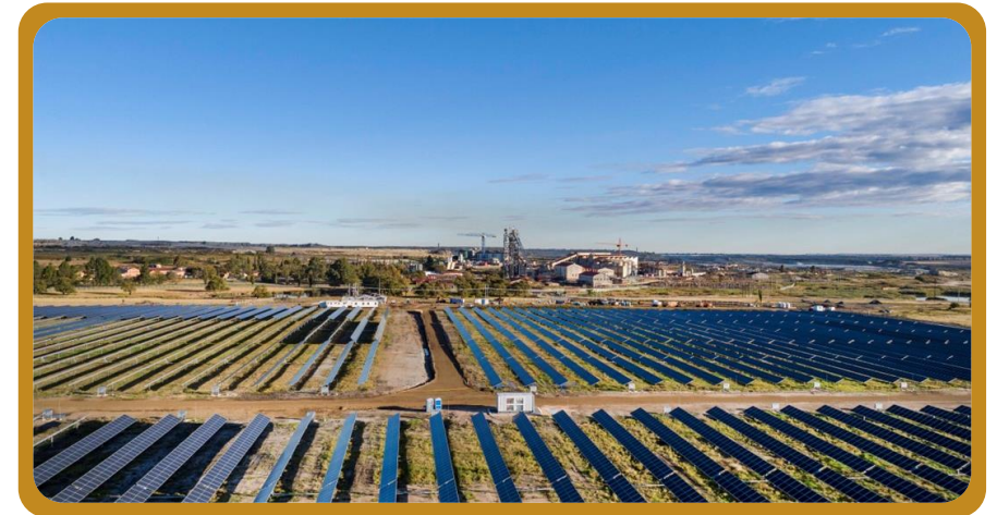
Solar PV plant at Evander Gold Mine
