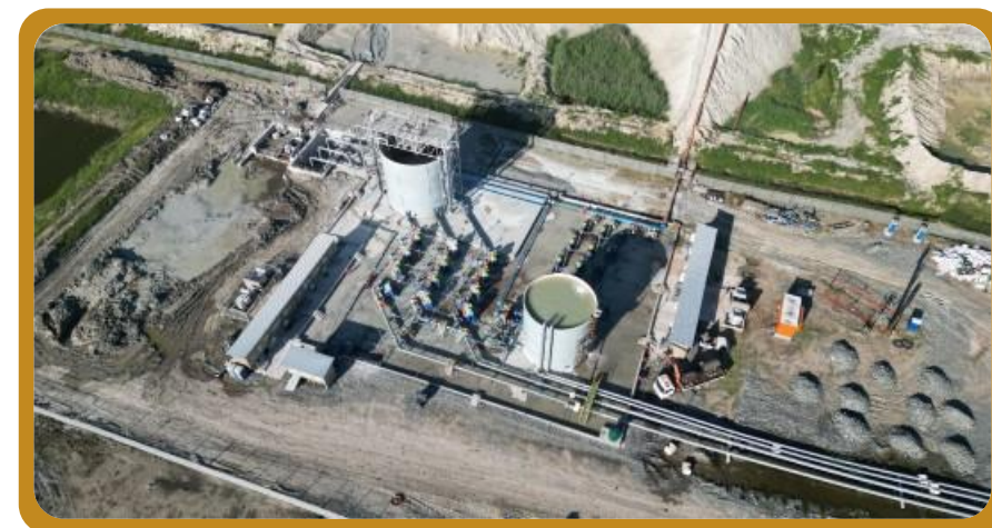
Completed Leslie/Bracken pump station at Elikhulu
