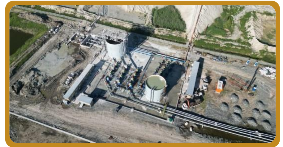
Completed Leslie/Bracken pump station at Elikhulu
